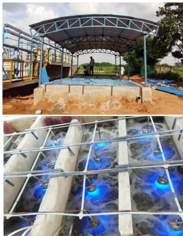
Figure 3. Pilot-scale anaerobic-aerobic algal-bacterial suspended-growth reactor, showing the LED-illuminated chamber where algal photosynthesis supplies the bulk of the oxygen otherwise provided by mechanical aeration.
